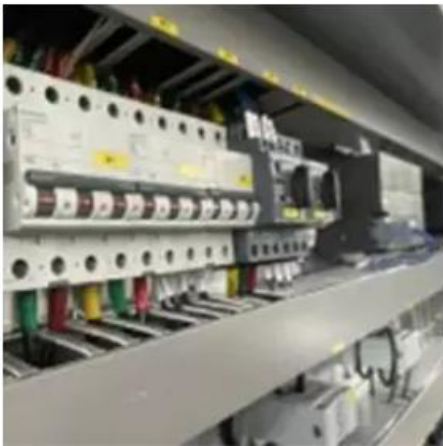
German Siemens electrical system
