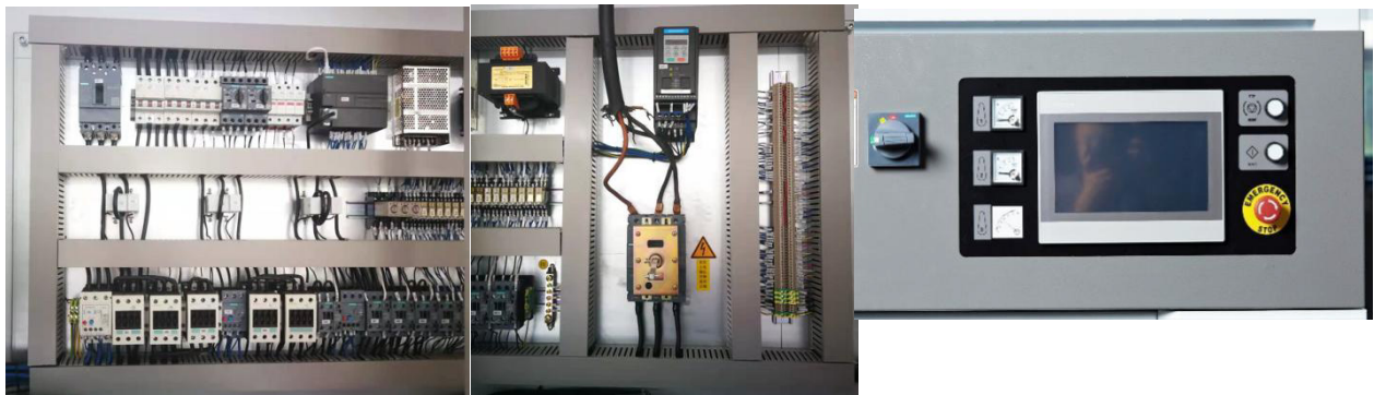
SIEMENS/ABB low-voltage Electrical parts
